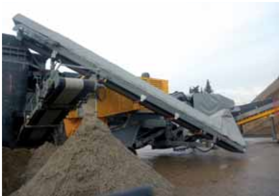
Photo: P1010701_hi.jpg / Text: The return conveyor housed for reducing the dust emissions.
